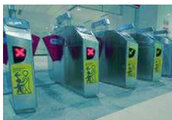
a ticket barrier
